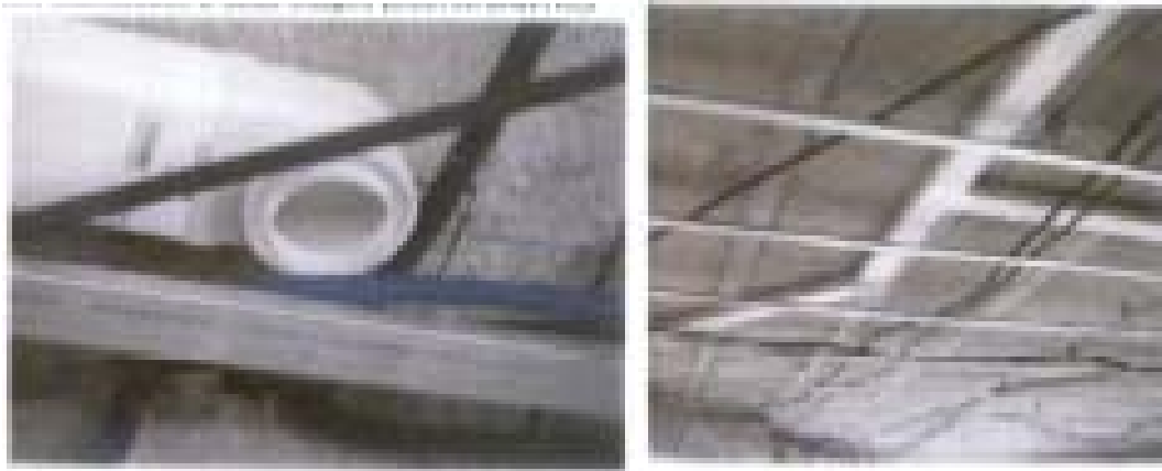
Figure 3-2: Example of ducts, Courtesy Atlantic- (CFP, 2006)
